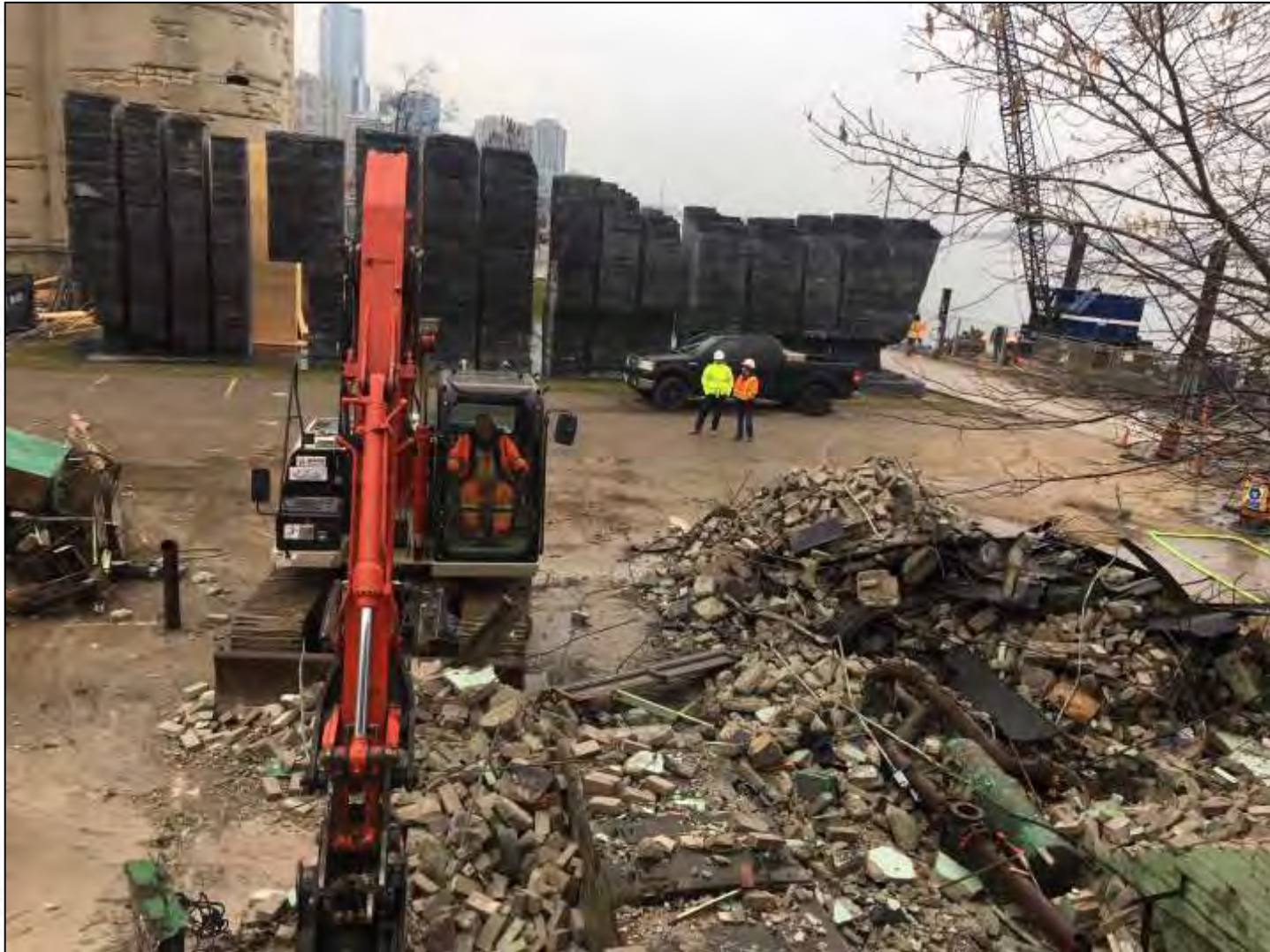
Fall 2019: Removal of former pump house, mechanical shed and abandoned subsurface utilities
