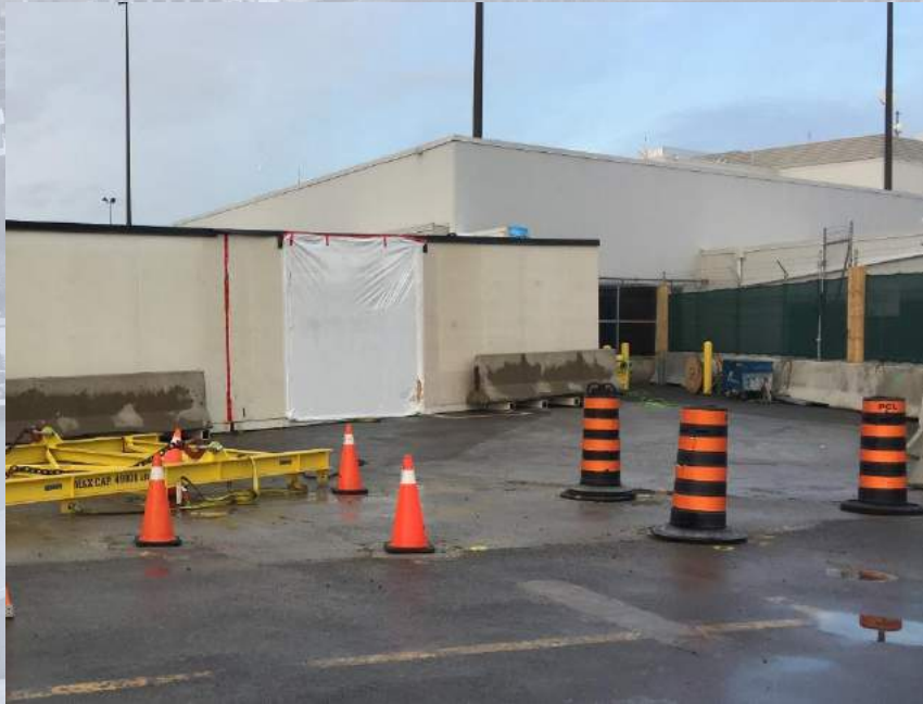
Module Temporary Gate in place
